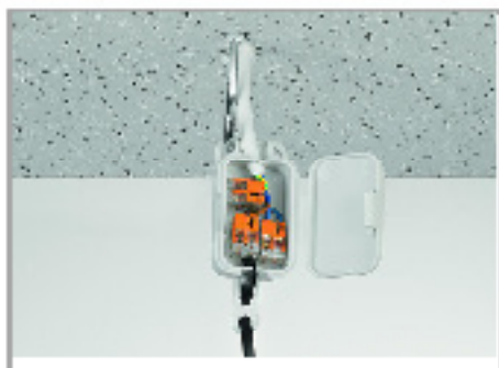
Pendant light connection in suspended ceilings
