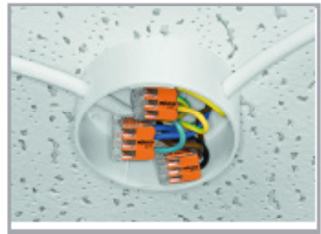
Lighting distribution in ceiling canopy
