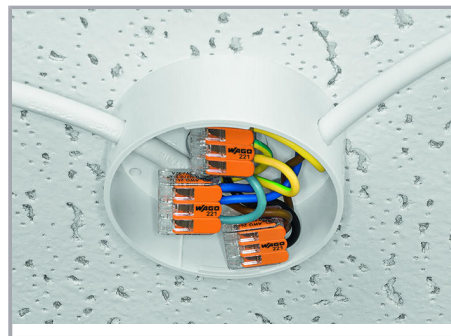
Lighting distribution in ceiling canopy
